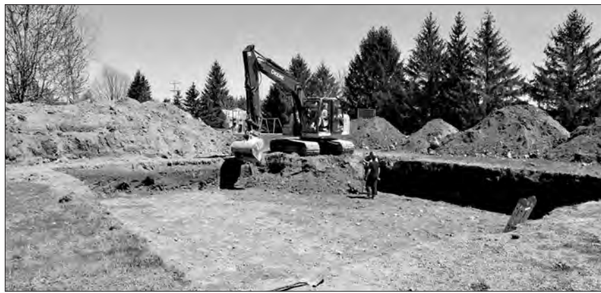
The foundation for Habitat for Humanity Cornwall and the counties' Winchester Springs home build project was excavated on May 9. Located in the Municipality of South Dundas, the new build is set to become the Rumohr-Boisvert Family's home before the end of the year. Casselman Photo
