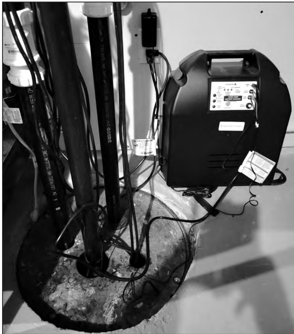
Pictured here is a recent Jason Munro Heating sump pump setup with a sealed sump pump pit with two pumps and one battery backup pump (three total). Courtesy Photo
