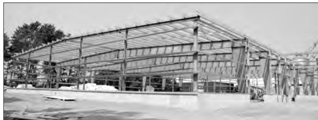
In this photo the skeleton of the new processing facility at the Sandy Row Sevita location has been completed. This was back in August of 2021. Morin Photo
