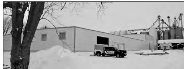
Construction of the new plant is just about finished as January comes to an end, with all of the processing equipment in place. Morin Photo
