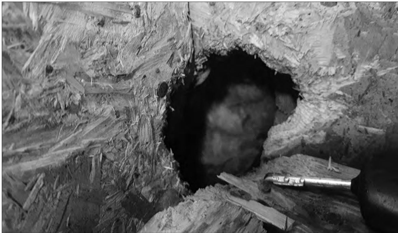
Rodents gnawed an interior wall (about 5" opening) to make their way into the attic in an Ottawa house in September 2021.
