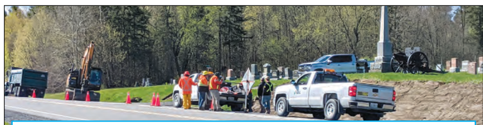
A portion of the roadside in front of Memorial Hill Cemetery near Lunenburg is prepared for planting by members of the SDG Butterflyway Project by a crew from the United Counties of SDG.
