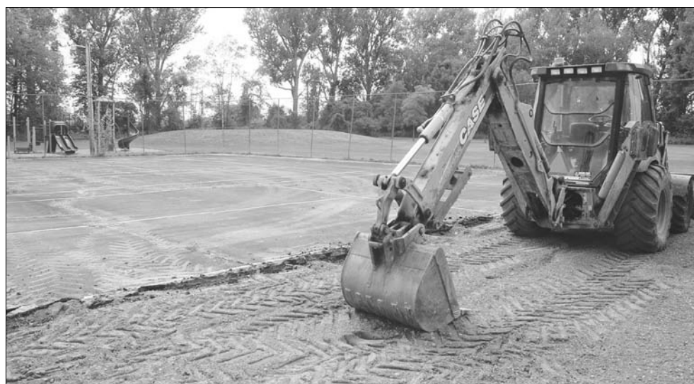
Work has already begun on the tennis courts at South Mountain. The tennis courts in Chesterville will have to wait until next year for their renovations. Morin photo
