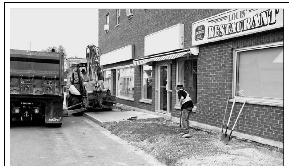
Out with the old in with the new D-Squared Construction Ltd. started the work of replacing some of the sidewalks in Chesterville on Wed., June 24. They planned for one day to remove the existing sidewalk and another day to pour the cement for the new one; this crew worked on King Street. Morin photo
