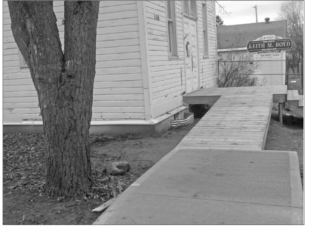
The Country Christmas show on Dec. 15 will be moved to the Youth Centre behind Russell High School due to ongoing construction of a wheelchair ramp at Keith Boyd Community Museum.
